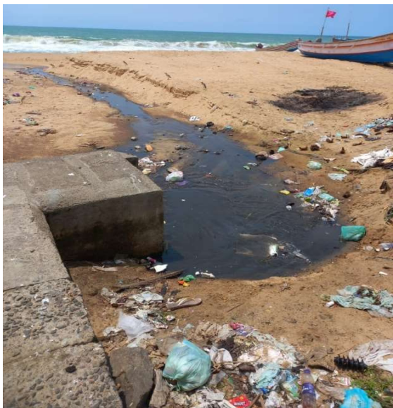
Greywater stagnation near sea
