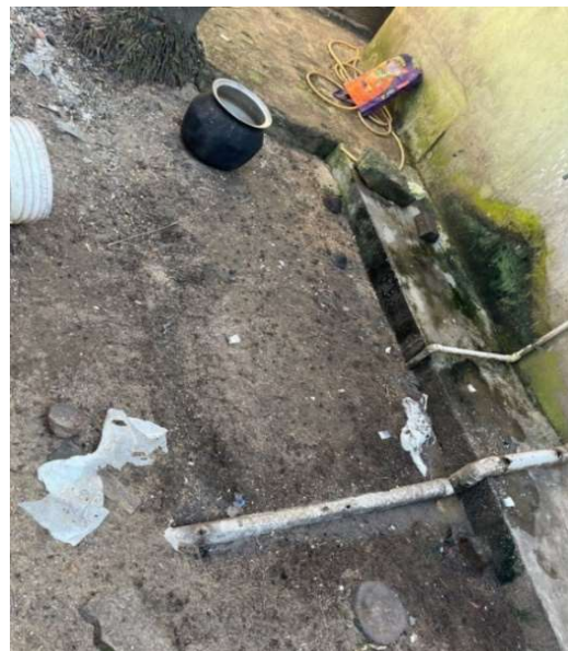
Greywater discharge to soil
