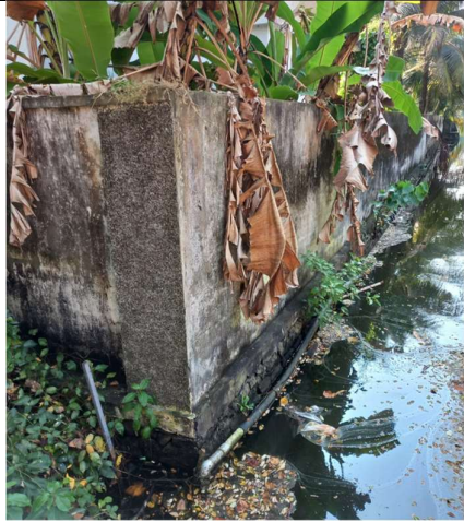
Greywater stagnation near house compound
