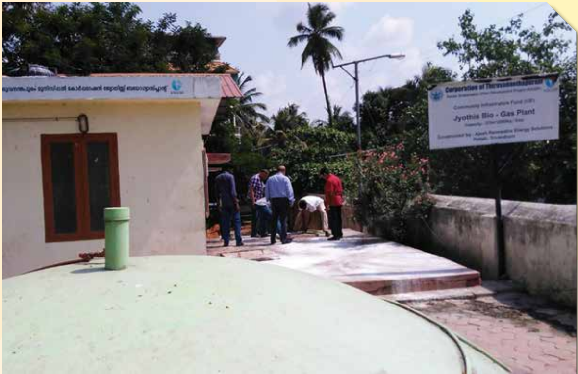
Biogas plant at Health Circle Office, Trivandrum Corporation Office Manacaud
