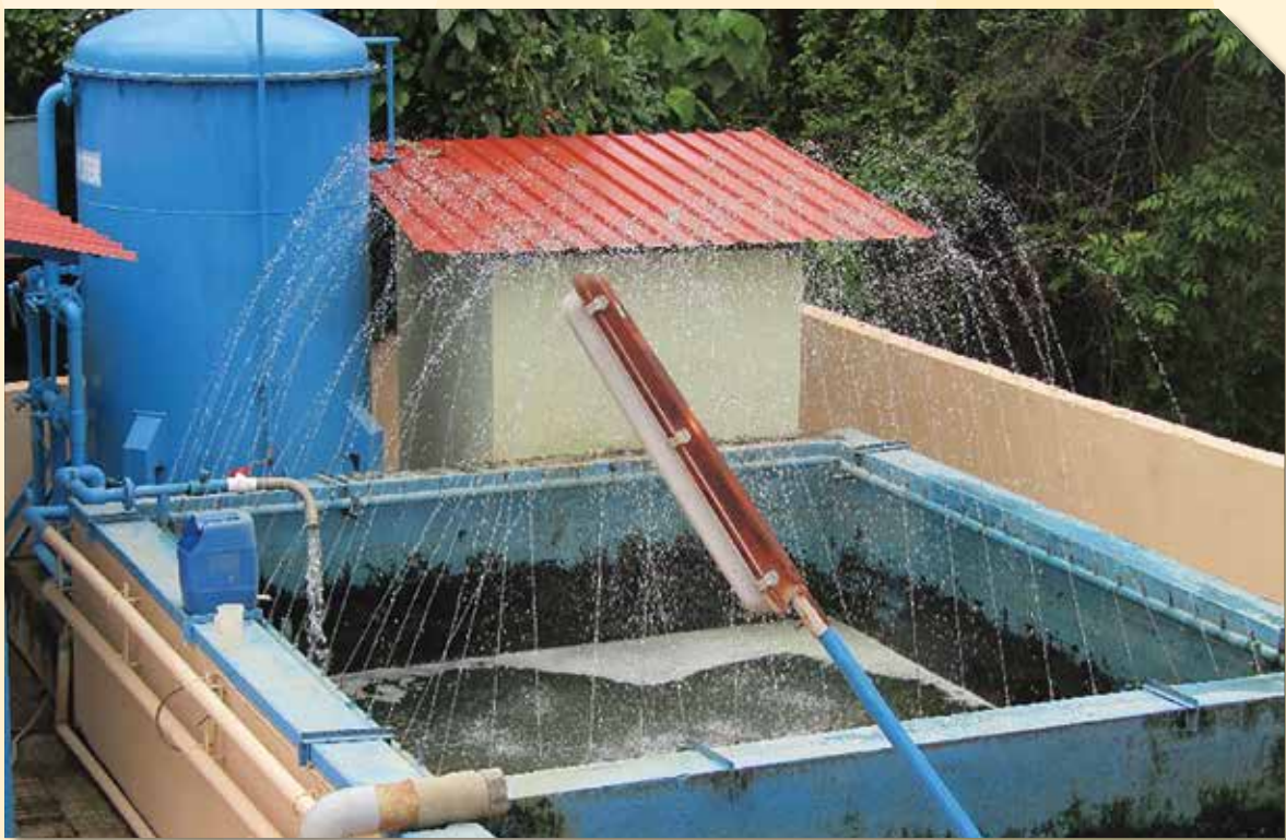
Sewage Treatment Plant, Taliparamba, Kannur
